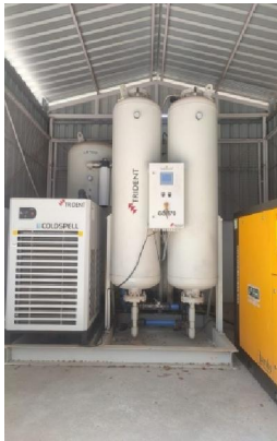
Oxygen Generator Plant
